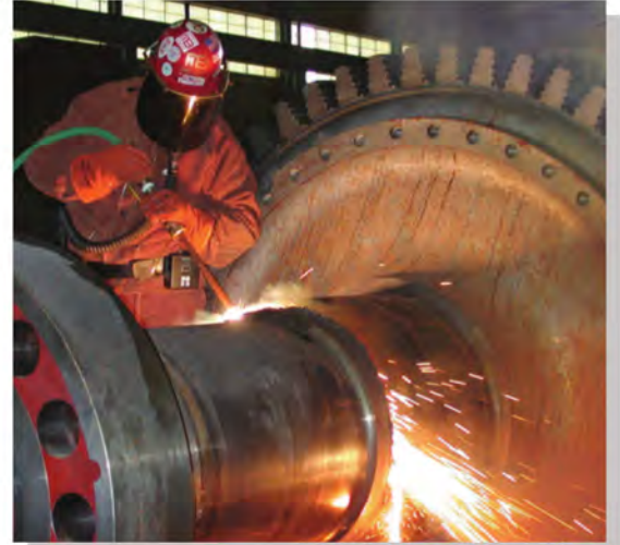
Complete demolition of Nuclear Power Plant Cutting steam turbine shaft 26 inches thick.
